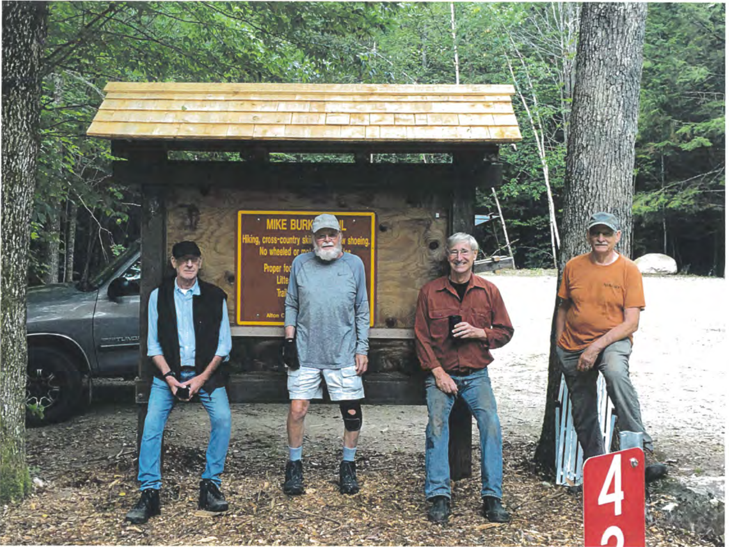
Kiosk repair and installation volunteers (L to R) – David Mank, Earl Bagley, Gene Young, Dana Rhodes, Russ Wilder (behind the camera)
